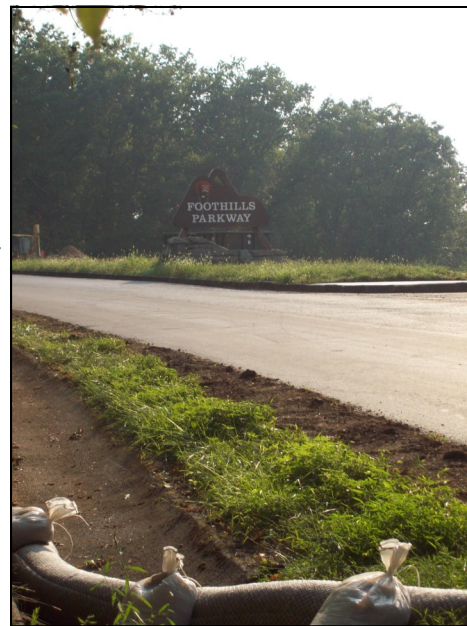
Last Fall, the U.S. National Park service used GeoHay to prevent erosion along a six-mile section of the Foothills Parkway in the Great Smoky Mountains National Park that was undergoing resurfacing.
